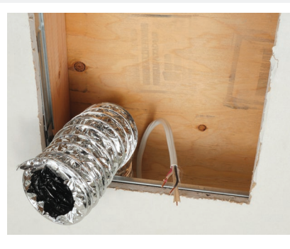
Existing 3" Duct and wiring
