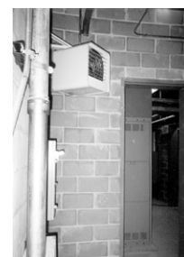
Freeze/moisture protection in a generator vault
